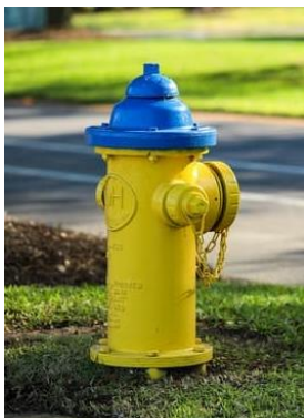
Figure 32. NFPA colour-coded hydrant.
