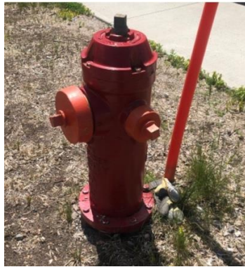
Figure 33. Hydrant located in the City of Dryden (source: drydennow.com).
