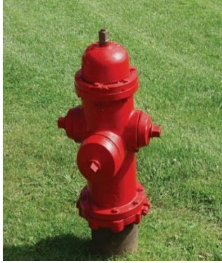
Figure 34. Example of a private fire hydrant.
